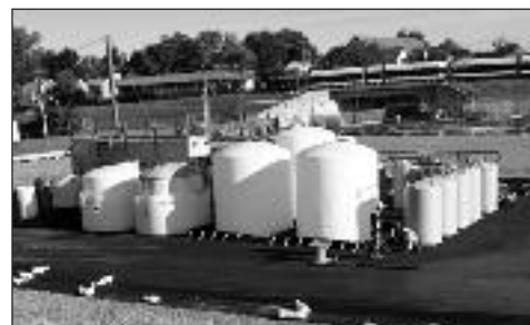
Water treatment system is located on portion of Garfield Avenue Site where chrome waste has been dug up and hauled away.
